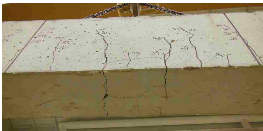
Figure D-12. Crack Pattern of Specimen BWOC-60 (Bottom View)
