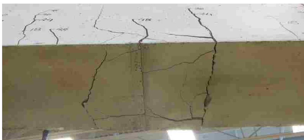
Figure D-24. Crack Pattern of Specimen TWOC-70 (Bottom View)
